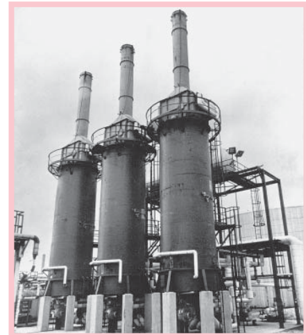
Liquid Asphalt Heaters
